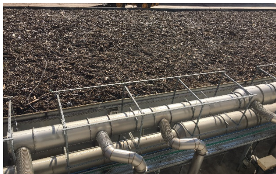
(3) BIOFILTER FOR THE PROCESS ODOURS ABATEMENT
